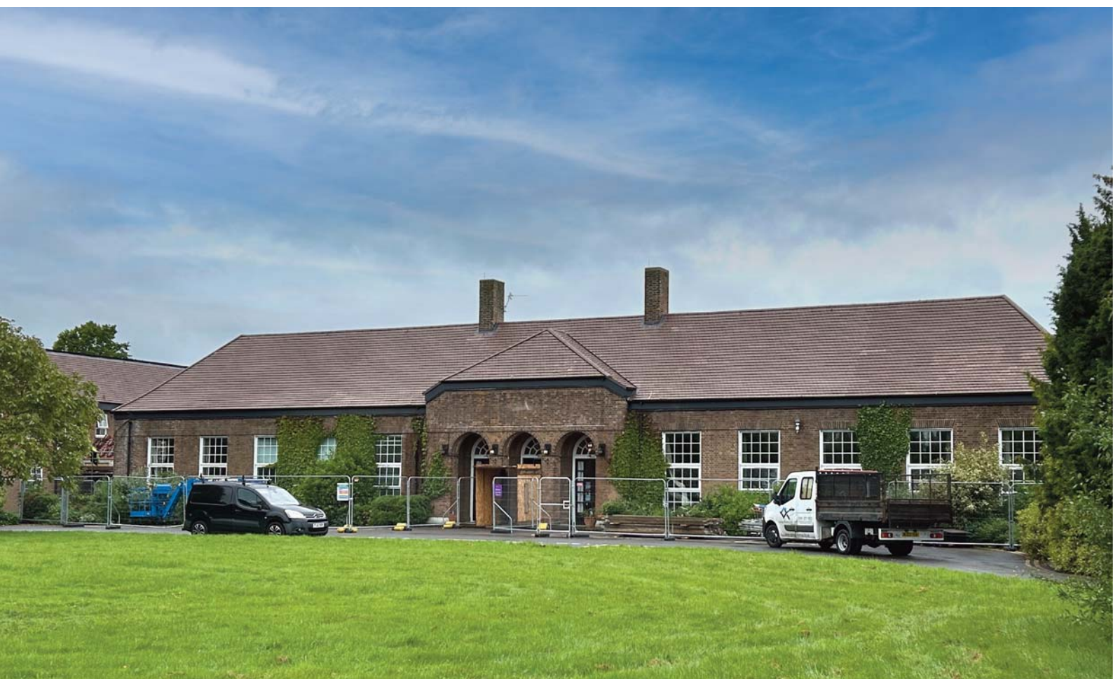
Springs Roofing Ltd - CLC, Officers Mess including east and west wings, RAF Leeming
